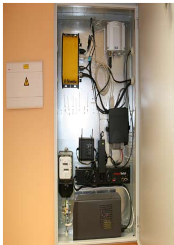
Fig. 2. LitPOS station with Trimble NetRS receiver
